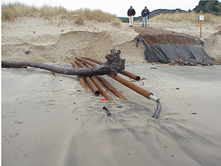
Figure 2-1. Cable landing infrastructure exposed by coastal erosion in the Rockaway Beach, Oregon area in late 2001. Image source: J. Allan.
